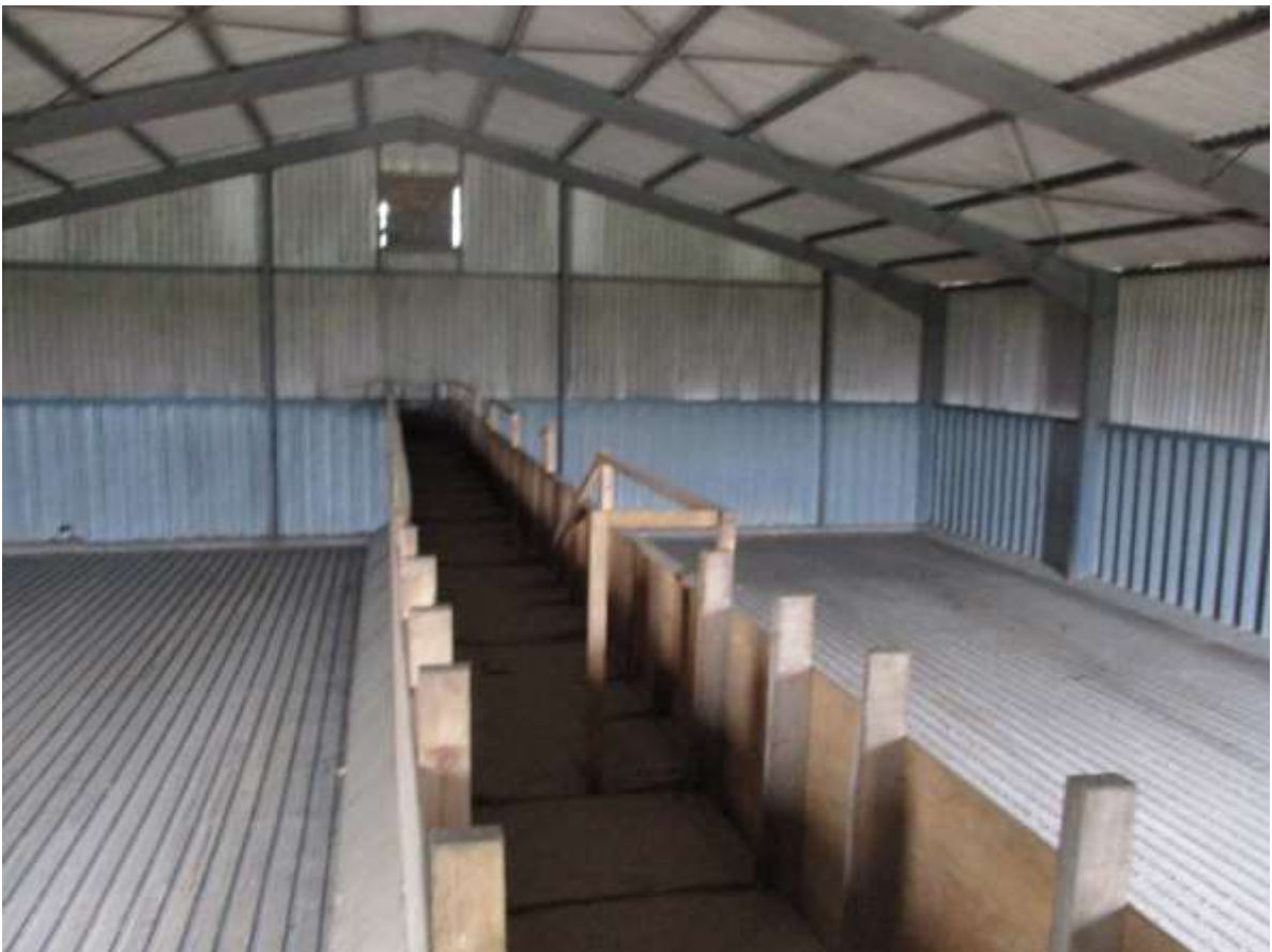
Plate 10: Central structure provides ducting to ventilate storage area.
