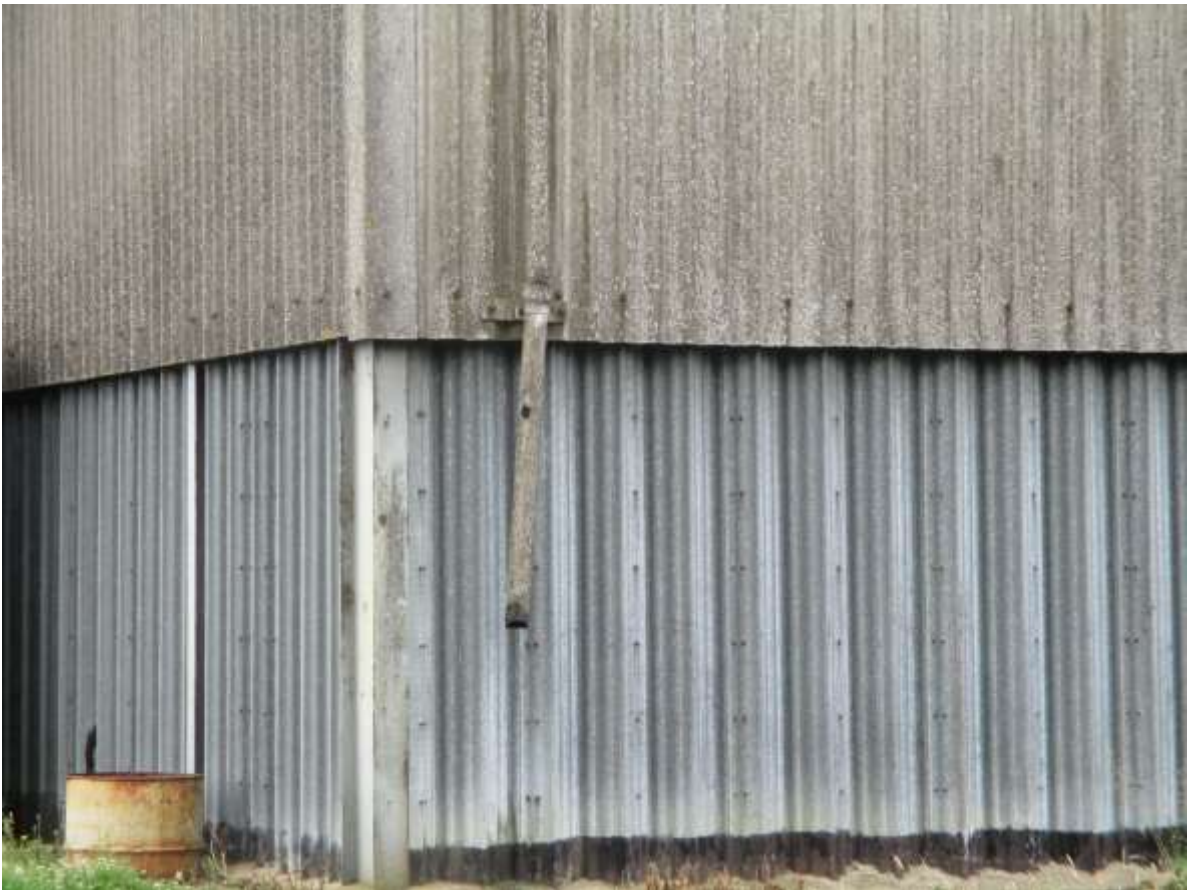
Plate 6: Sections of downpipe missing.
