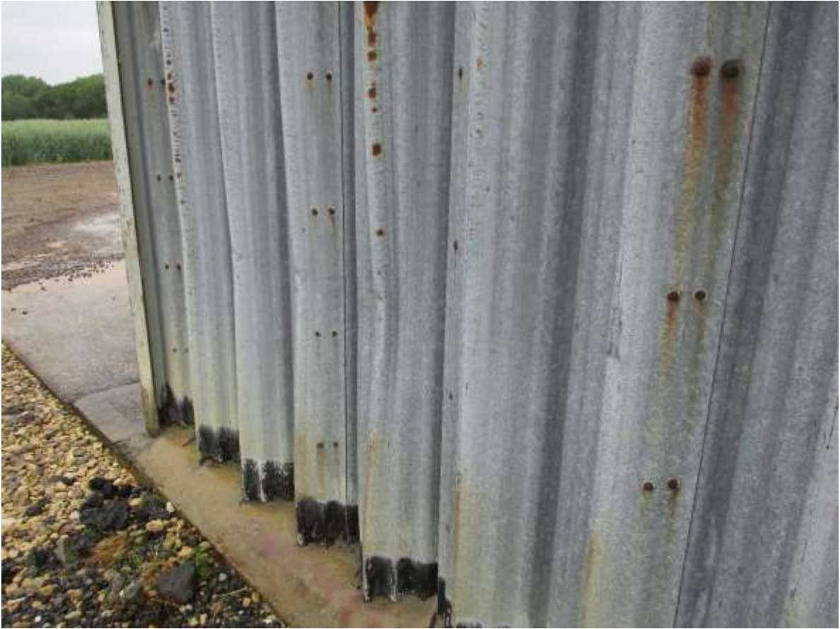
Plate 7: Minor cosmetic impact damage near front corner.
