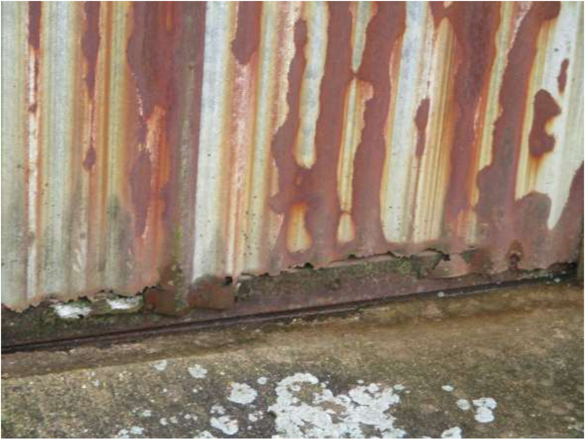
Plate 11: Wear and tear to the main front doors.
