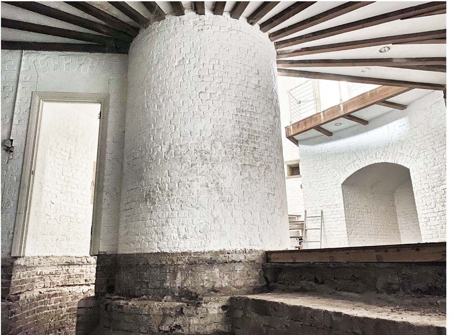
Lower level prepared for the installation of a new underfloor heated suspended slab.
